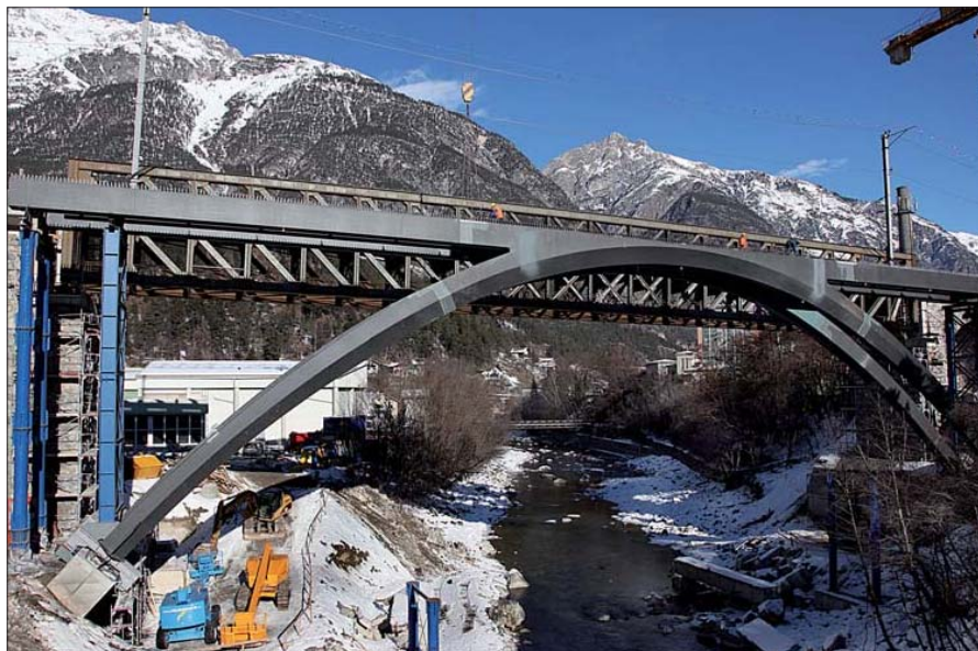
View of the new steel arch bridge in front of the existing lattice girder bridge, during construction
