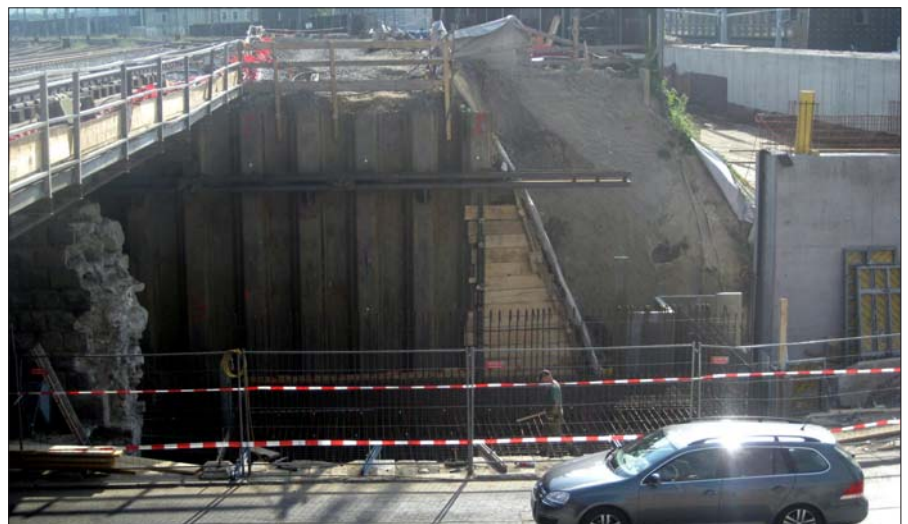
Railway bridge over the Friedhof Road, building pit for the establishing of the bearing structure no. 3
