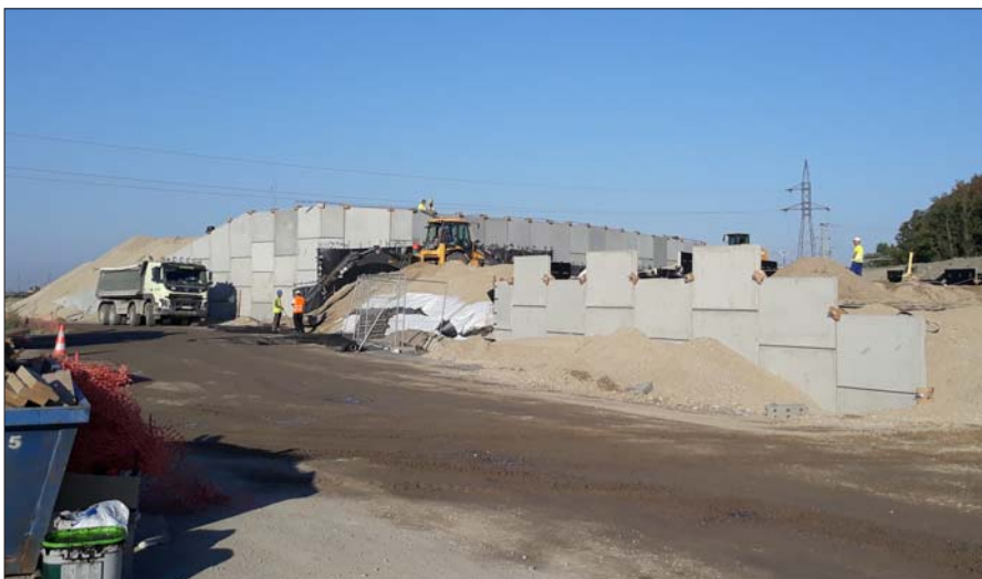
Construction of bridge abutments by reinforced soil with a facing of concrete panels
