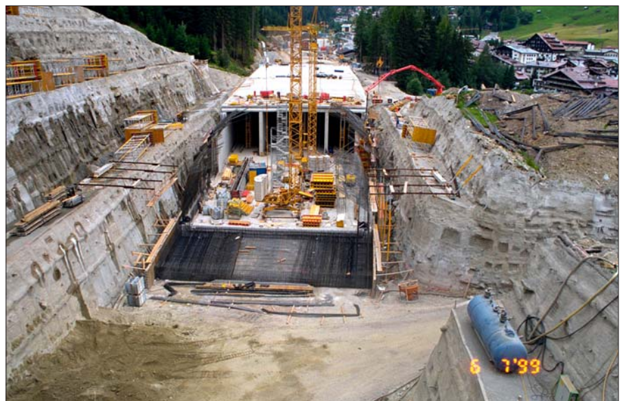
Area of the cut and cover method Wolfgruben Tunnel (View towards the west)
