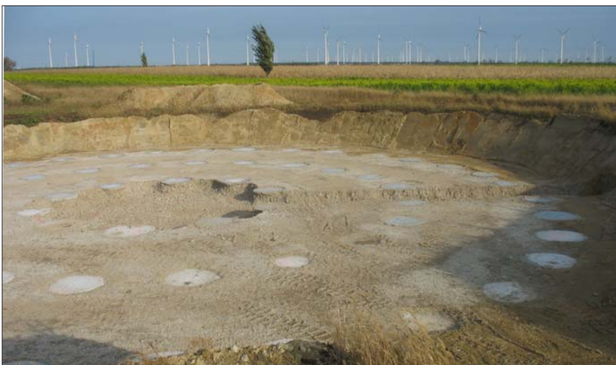
Prepared contact surface after soil improvement by means of grouted gravel piles
