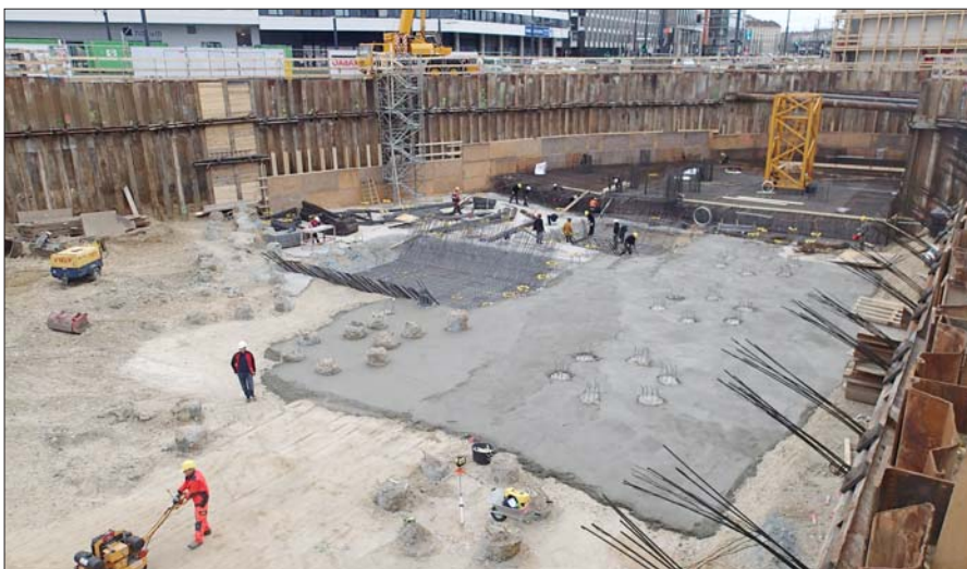
View into the construction pit; At the left edge of the picture excavation area of the sealing wall for the tar pit remediation
