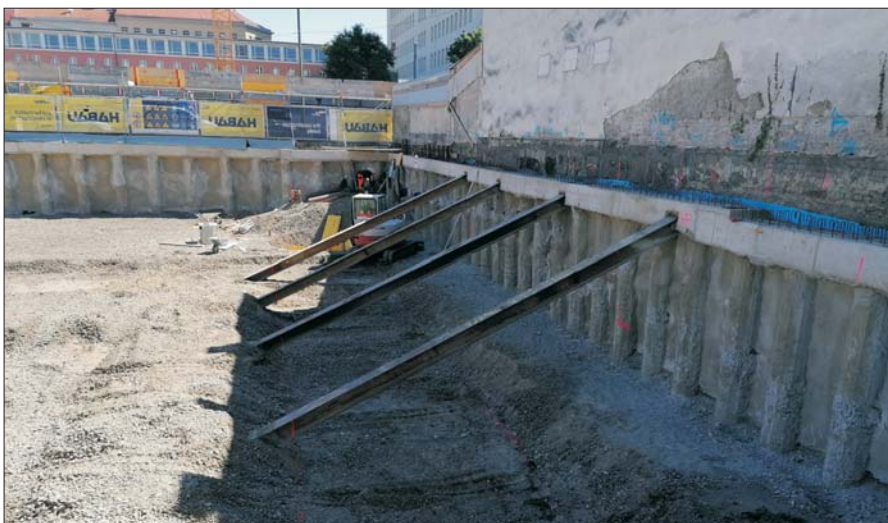
Building pit support system and underpinning of the existing building by intermittent bored piles
