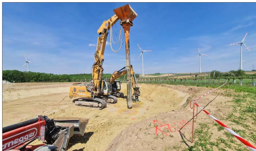
Underground improvement by means of vibro-displacement compaction at the Wind Park Trautmannsdorf
