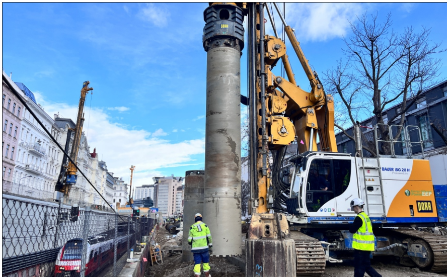
Construction of bored piles between Rennweg stop and Vienna Central station (four drilling rigs simultaneously)
