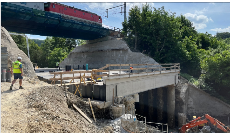
Construction of the underpass of the road L123, Phase: excavation between bored piles
