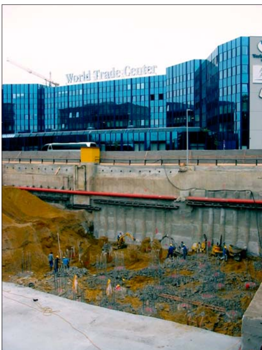
Excavation to maximum depth (top of the circularly arranged bored piles for the tower foundation visible)
