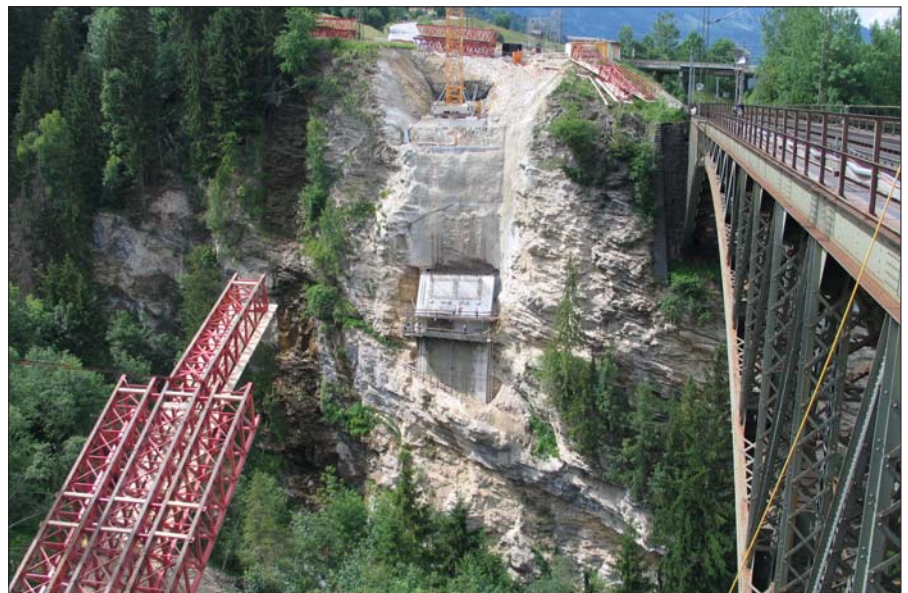
View of the Anger Gorge Bridge, existing and new (under construction); View towards abutment side Schwarzach
