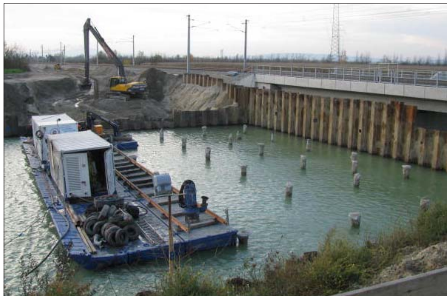
S1 underpass of the Northern Railway Line, Construction of the concrete floor below ground water level
