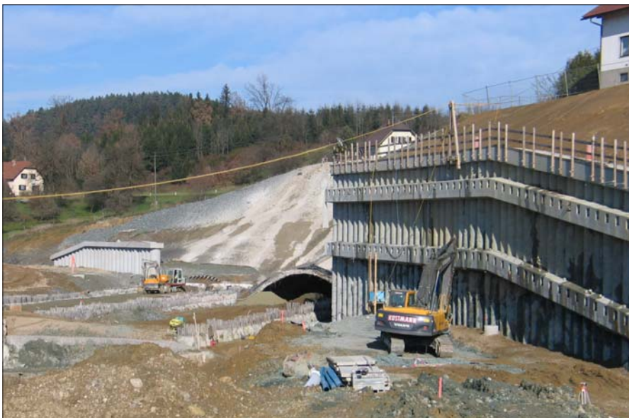
View of the southern portal of the Koralm tunnel; on the right anchored bored pile wall upward the track of the regional railway
