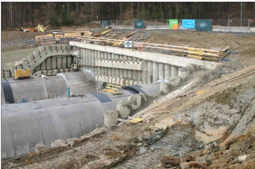
View towards the eastern portal of the Koralm tunnel (portal wall of the tunnel with closed advance)
