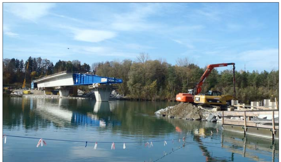
Establishing of the Bridge across the Drau river by Incremental Launching Method
