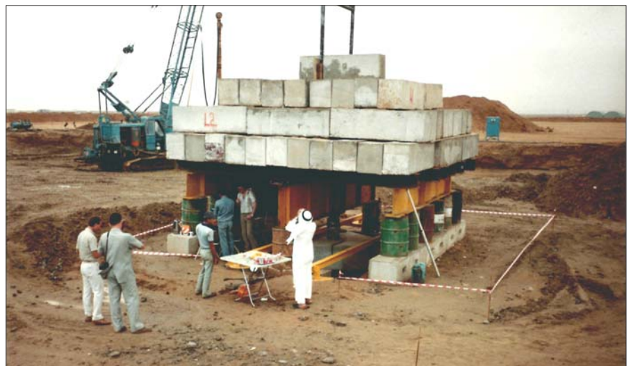
MTTS, Pumping Station 1: Test load of the subsoil improvement by means of gravel piles
