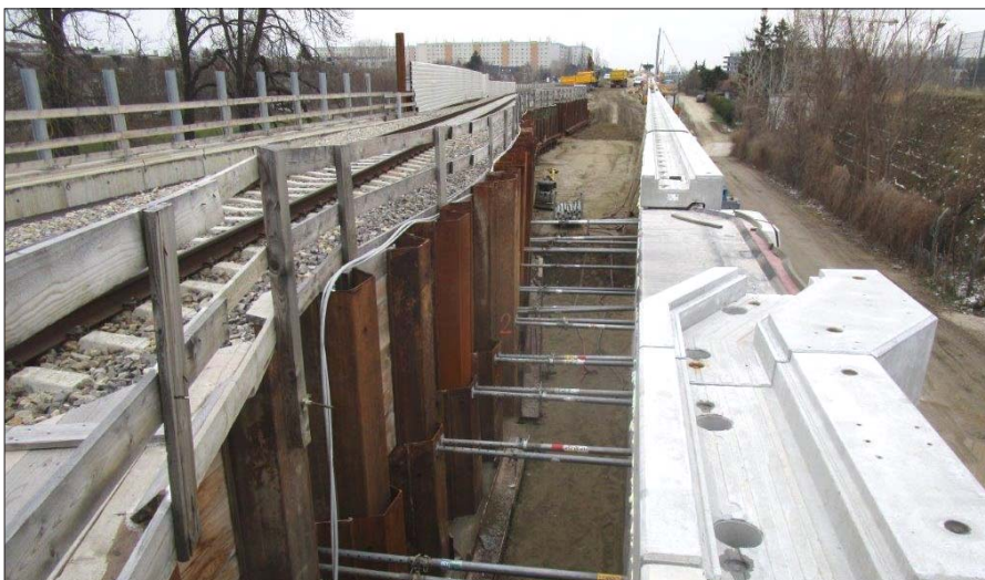
Sheet pile wall during the construction of the retaining wall between Auparkweg and Hirschstettner Straße
