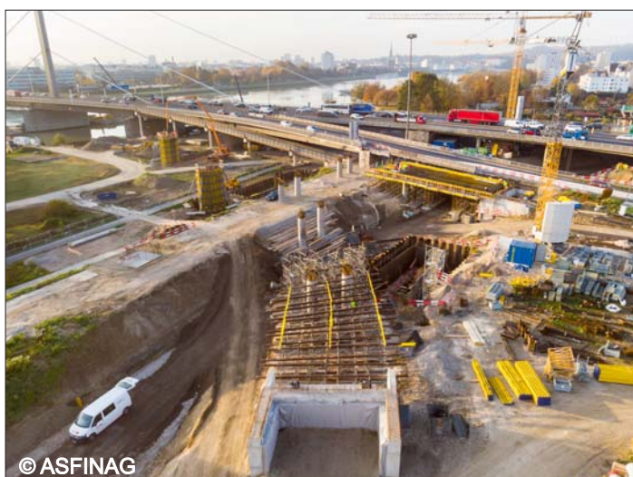
Setting up of the ramps for the by-pass bridges across the Danube
