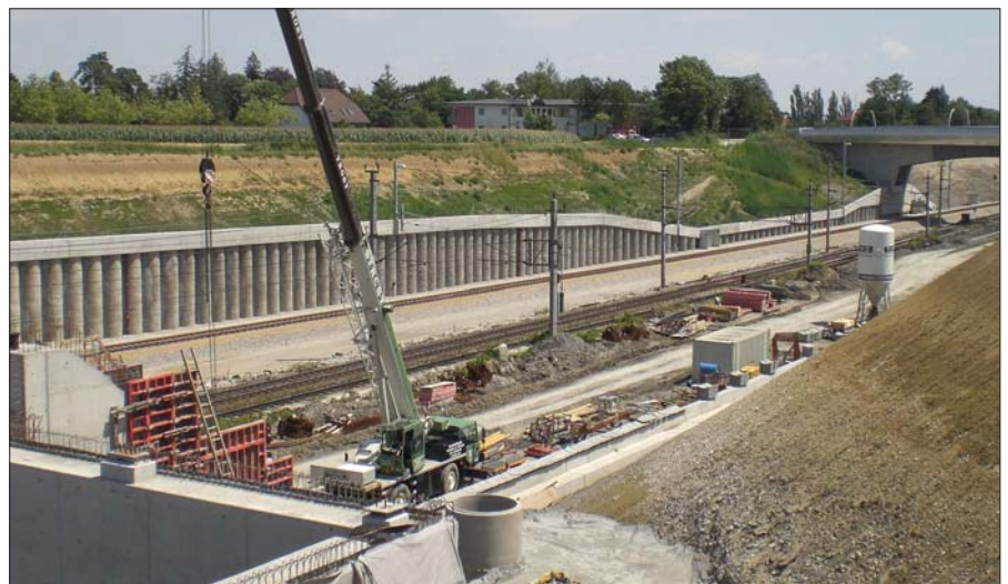
Cut at the western section (view towards east), retaining structure in form of an intermittent bored pile wall
